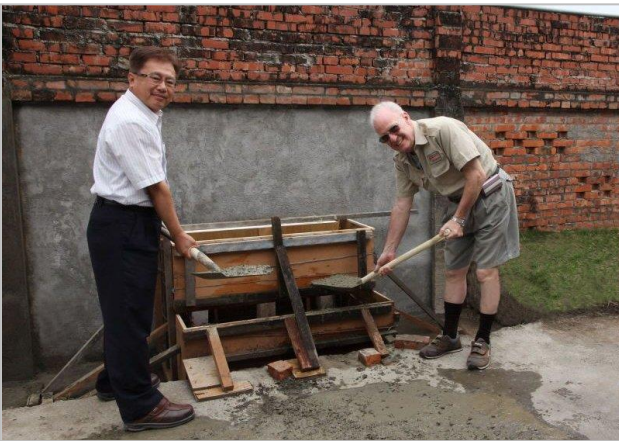
With Mr. Shieh MOEA, shoveling the first cement into the new Taichu Memorial base.
